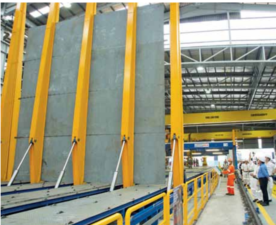
The panels are now turned using a flip-over machine and moved from station to station using a conveyor system
