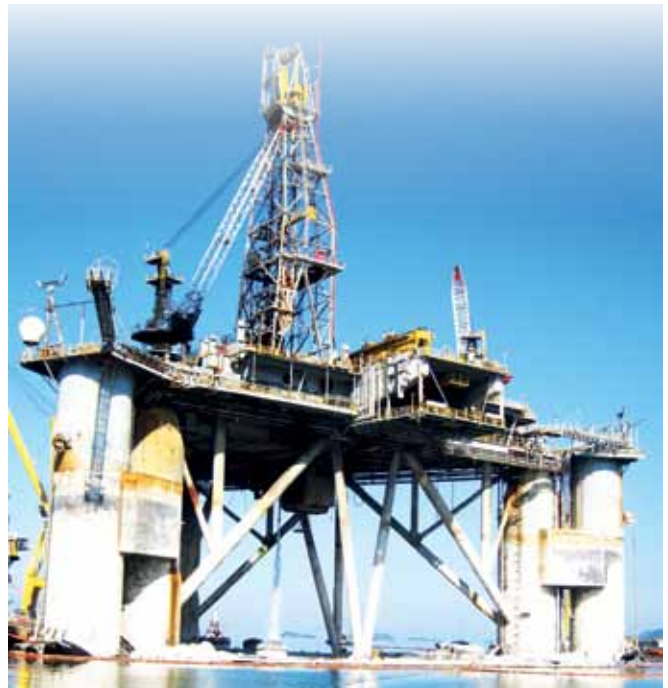
Noble Drilling commended BrasFELS for completing the repair and modification of Noble Paul Wolff safely and promptly
